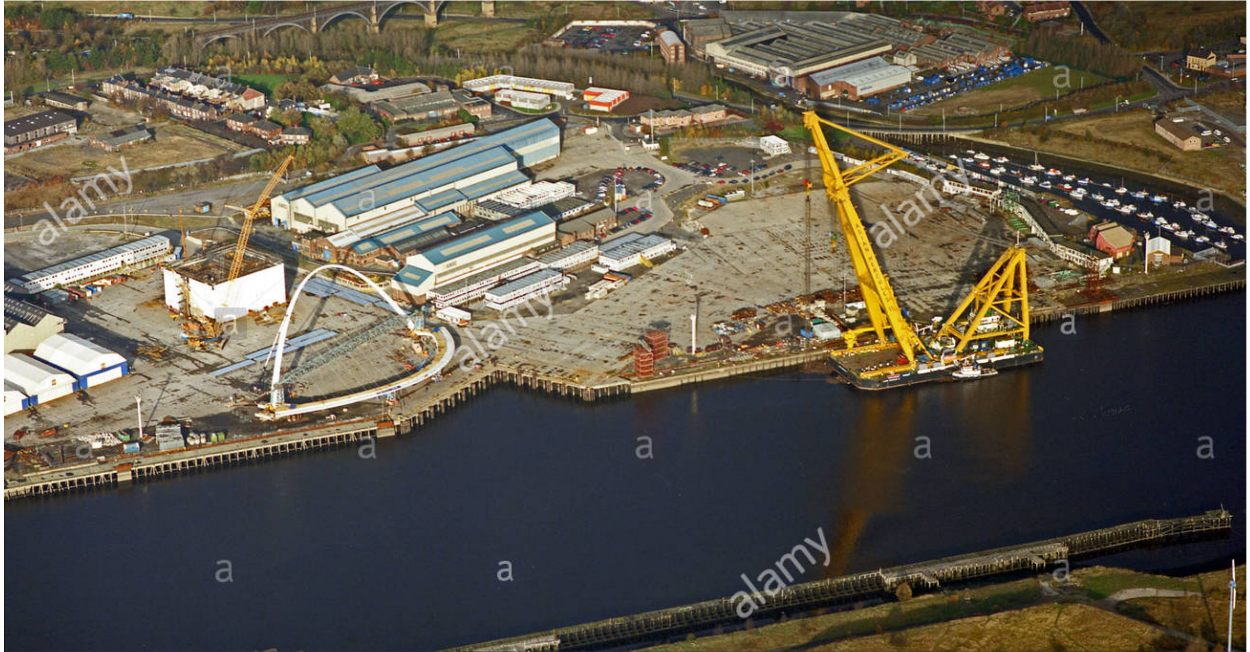
Fabrication of the Gateshead Millennium Bridge takes place offsite: Bridge completely prefabricated and shipped to site.
